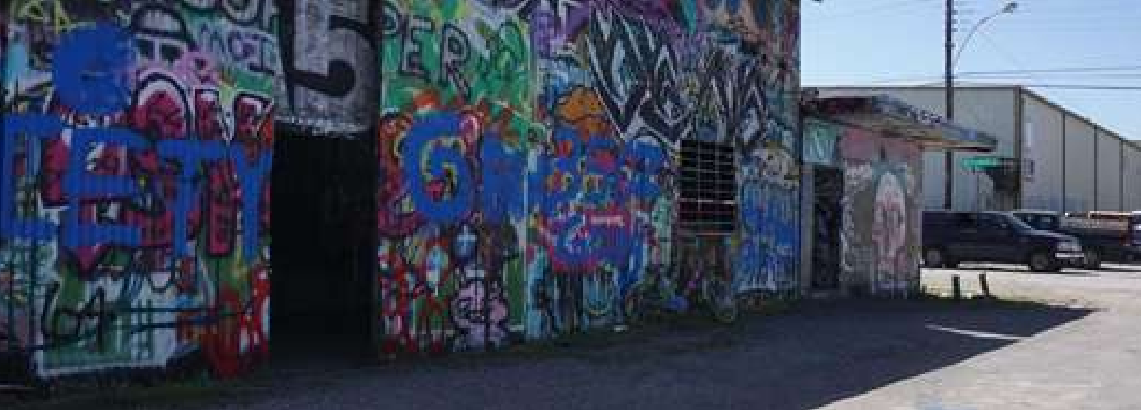
Example of Graffiti on local buildings — taken during a ride-along with Code Compliance. Image Credit: Justin Childress
